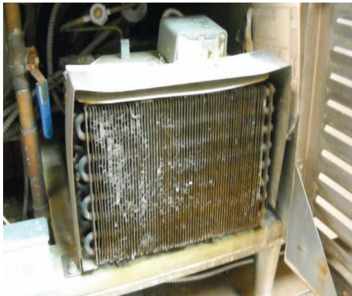
This old and tired unit stands in contrast to the other example pictured above. It is not operating efficiently, wasting hundreds of dollars a year in electrical consumption. It is only maintained a few times a year and is heading for an early grave.
