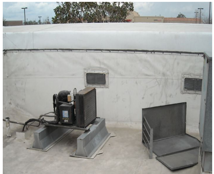
This unit was found with its condensing unit enclosure lying on the roof. A rainstorm blew the cover off and damaged the fan motor, resulting in a service call.
