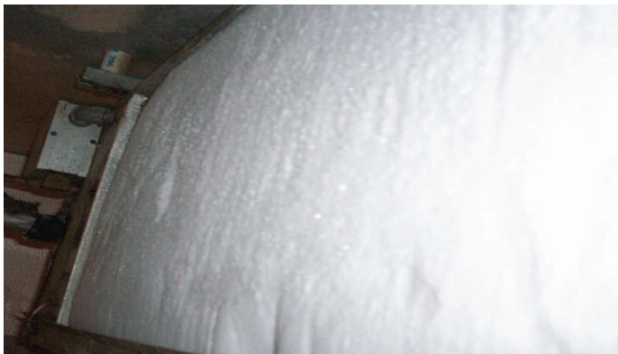
During a routine maintenance inspection, we discovered the evaporator coil in this walk-in cooler was a solid block of ice. The thermostat control was turned down to 25 degrees from the 35 degrees set point, and the compressor was running continually for several weeks. The kitchen staff did not know the evaporator coil was iced up and hadn't noticed that the core product temperature had been well over 41 degrees for quite some time.
